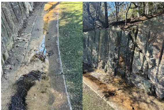
Photo: 1. Seeping from the rocks with the remnants of the heavy rains will need to be addressed in any future design
