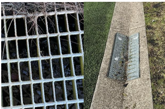
Photo: 2 Open grills allow microplastics and other rubbish access to the storm water system
